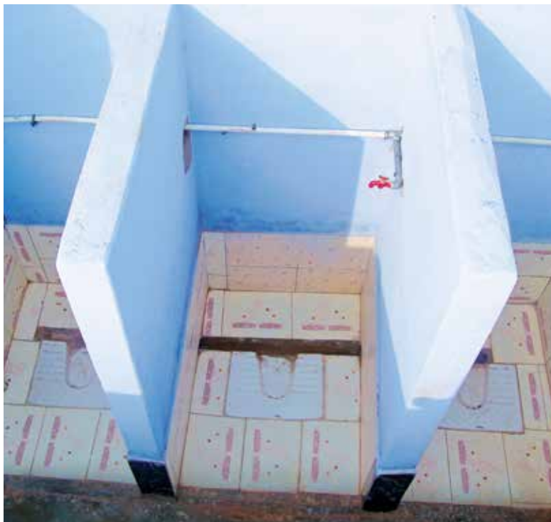
Running water inside the urinals ensures that the structure is well maintained
